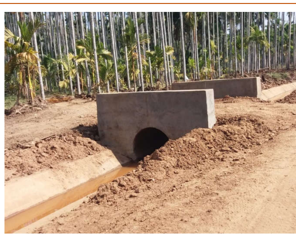
Pipe Cart Bridge
