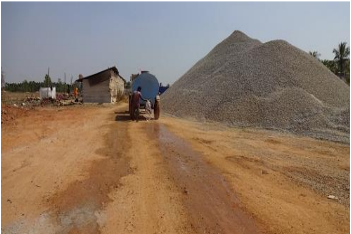
Contractor watering the Timlapura Campsite to prevent dust generation-unannounced visit by PSC to the campsite on 03.02.2016.
