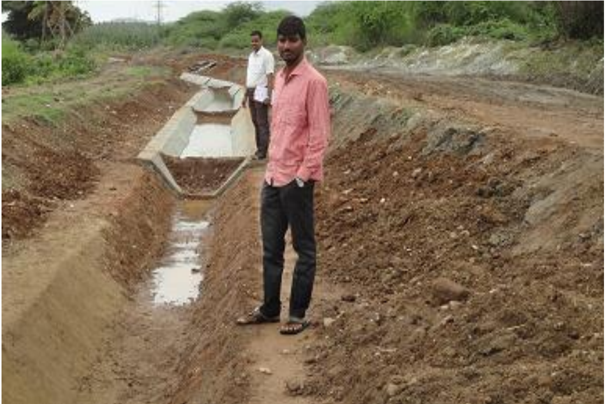
PSC Staff at the construction site to inspect the Silt Disposal Practices of the Contractor –June 28, 2016
