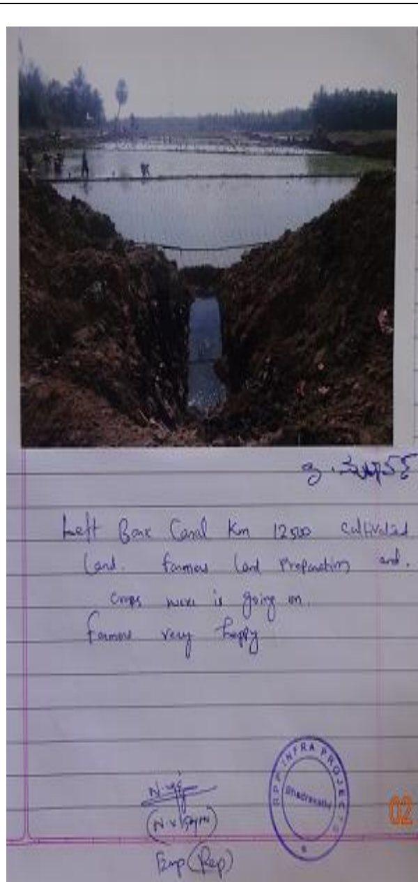
Farmers acknowledging that their routine work is not being hindered by the Contractor during the rehabilitation work
