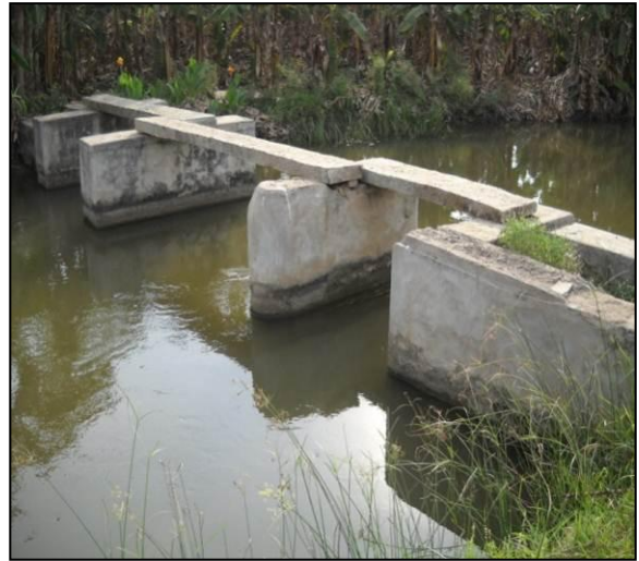
Fig 13.10 – Poor crossing structure
