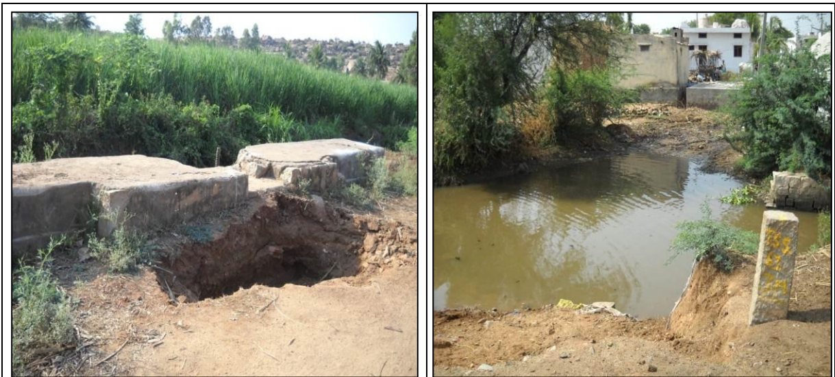
Fig 13.5 – Damage due to seepage and poor maintenance
