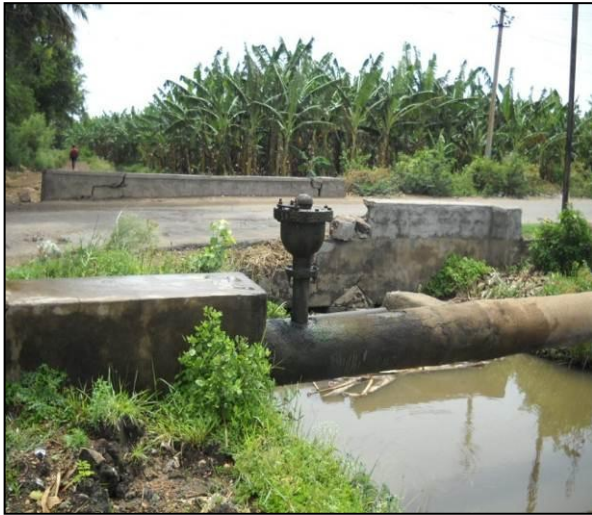
Fig 13.9 – Damaged Service road
